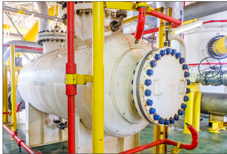
Figure 2: A test separator provides an opportunity to evaluate the output of each well pair individually.
