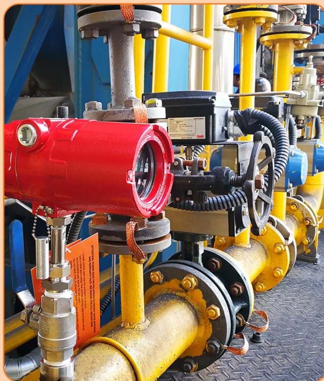
Figure 7. A thermal mass flowmeter was installed at a PTA chemical plant in China to measure methane waste gas.
